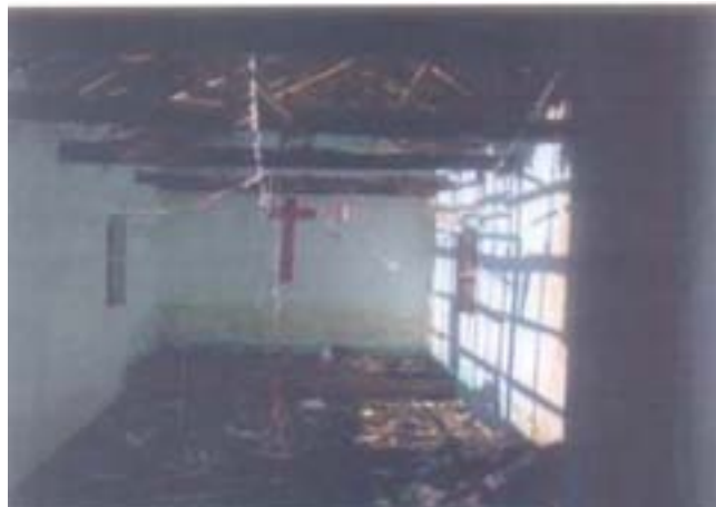
More than one hundred churches, presbyteries and convents were destroyed
